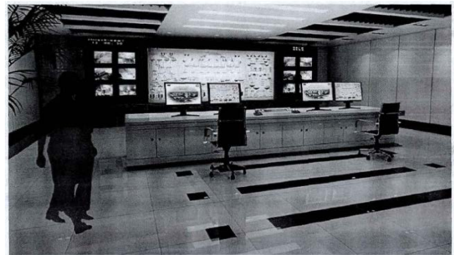
Fig. 10. System central control room.
